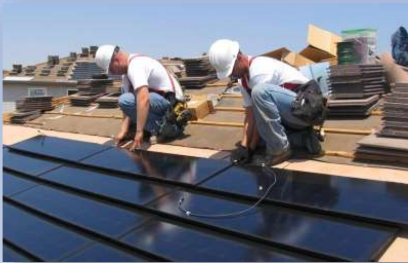
Zero Energy Community Rocklin, CA
